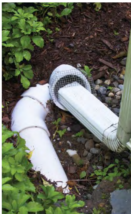
A partly buried drainage pipe attached to the downspout of a house helps direct stormwater away from problem areas.
