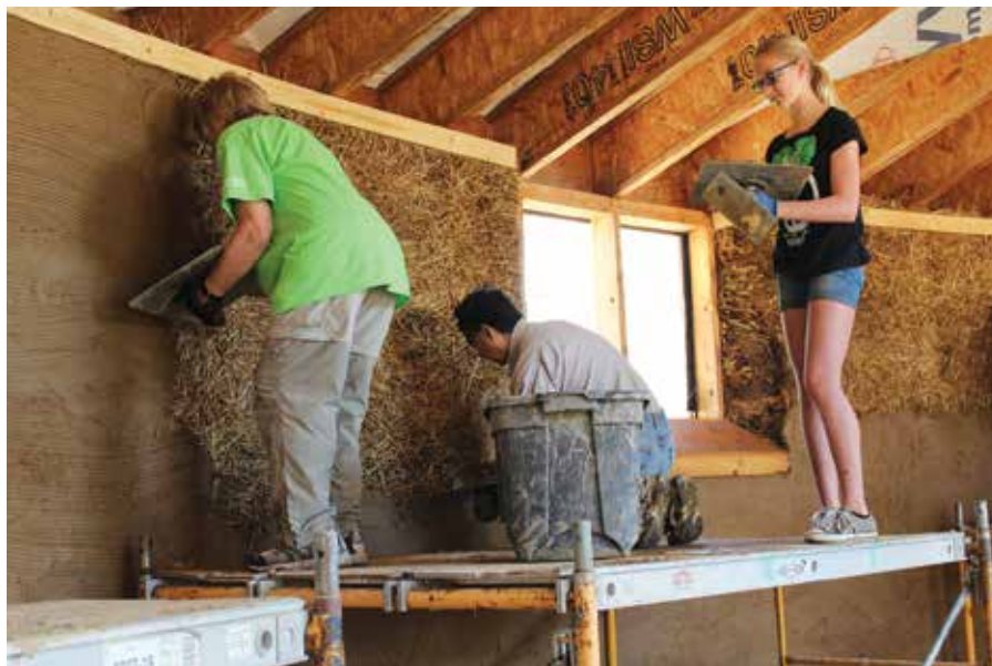
Spring Harbor Middle School's greenhouse features interior walls insulated with light straw clay.
